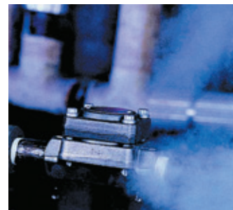
FIGURE 2 Defective gasket of this trap permits loss of live steam from the system.
